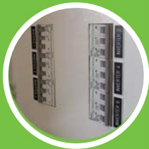
Circuit Breakers for Inverters
